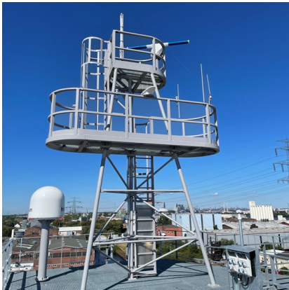
(b) Antenna platform on the roof of the building.
