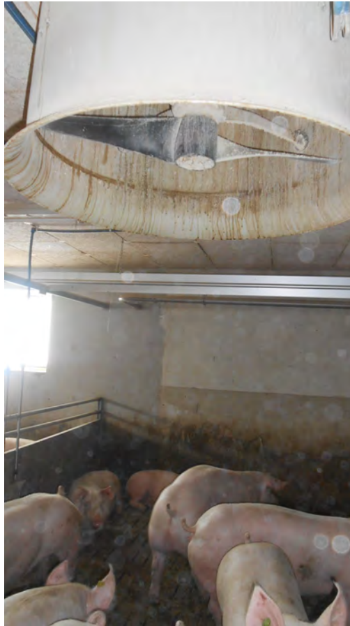
Figure 4-2 Example of emission extraction from a piggery. (Courtesy of Air Environment)
