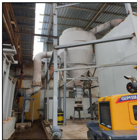
Fig.5. Discharge cyclone and hopper for dried material
