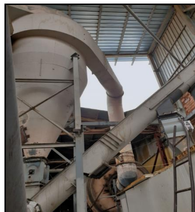
Fig. 6. Screw conveyor to hammer mill
