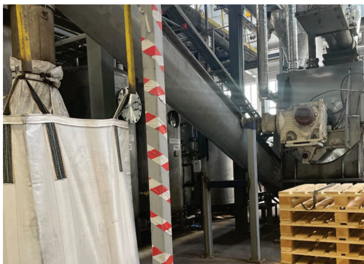
Figure 9: Continuous drying equipment for installed at ReSiTec
