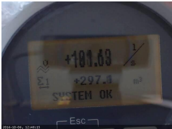
Figure 30: Example image of the display of the discharge sensor in pipe p1.
