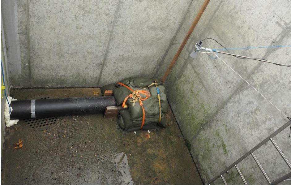
Figure 3: Pipe p6 in shaft s5 in which the flow meter p6_q&h_p_nivus is located. Ultrasonic water level s5_h_us_maxbotix_1 can be seen on the right.
