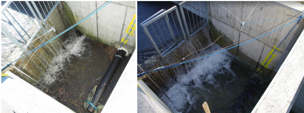
Figure 28: locations of ultrasonic sensor as s5_h_us_maxbotix_1 (left) and s5_h_us_maxbotix_2 (right). Pipe p6 is visible at the bottom of the shaft.
