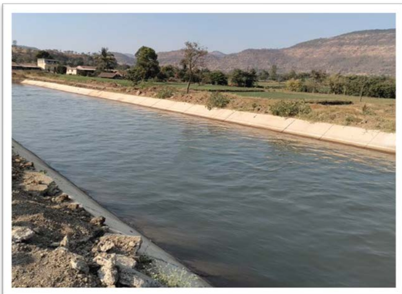
Irrigation canal in Dimbhe command area. Credit: Barbara Willaarts
