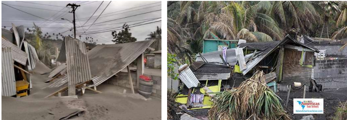
Figure 6.12 Damages to roof due to ash load. Source: NewsAmericaNow
