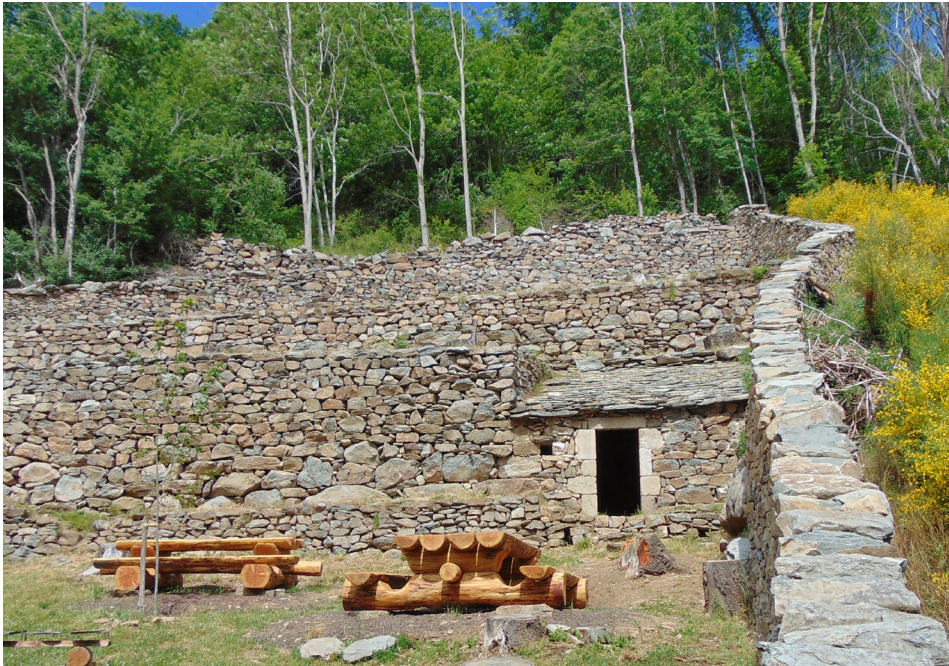
Figure 2. Stone hut for storing tools and products made of stone has been repaired (photo by Gérard Collange).
