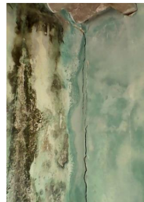
c) Interior weathering and damage (credit: J. Biles)
