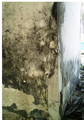
b) Exterior weathering and damage (credit: J. Biles)
