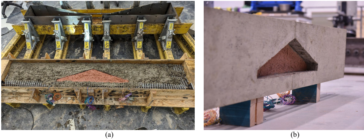
Figure 2: Manufacturing of test specimen (a) Inserting the reinforcement in stages after a layer of the functionally graded concrete had already been cast (specimen was cast sideways) and (b) tailored specimen after demoulding.
