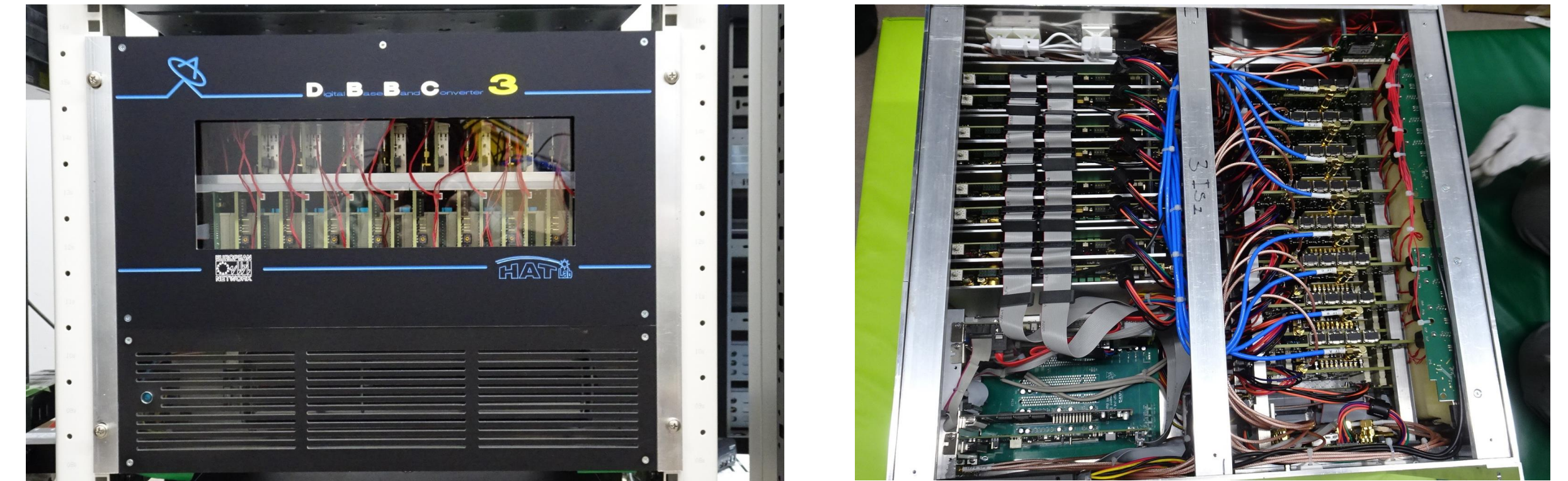
Fig. 4: (Left) Front view of the DBBC3 newly installed at the Ishioka station. (Right) Top-down view.
