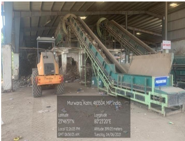
(c) RDF Processing unit:
