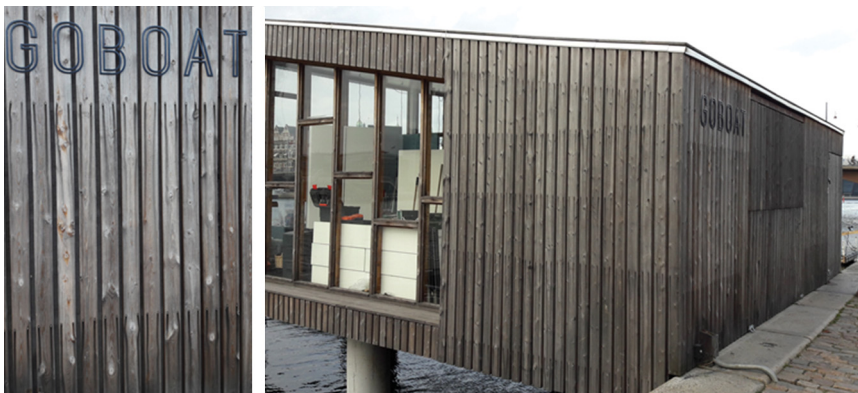
Figure 9.5 Furfurylated wood in service: a boat rental station in Copenhagen.
