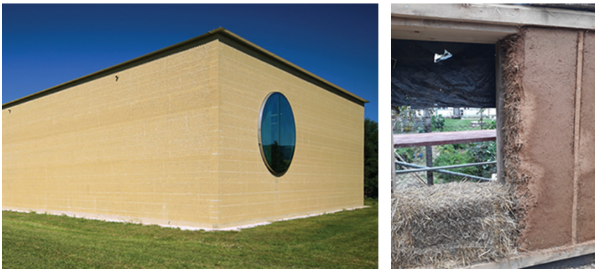
Figure 9.20 Rammed earth façade: Ricola storage and herb processing building, Laufen (architect: Herzog de Meuron, 1986–1991; left) and straw wall finish with the clay layer (right).
