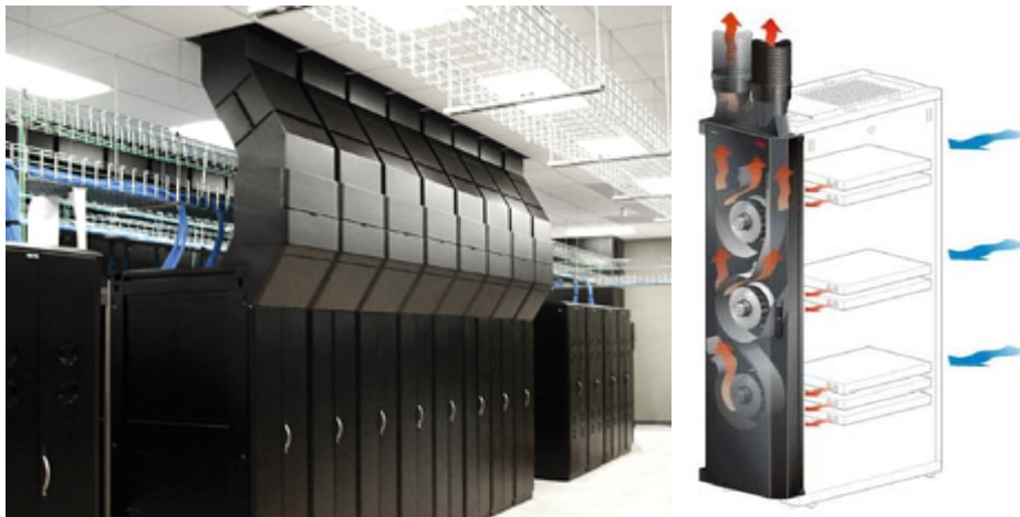
Figure 2 Server racks with dedicated exhaust chimneys h
