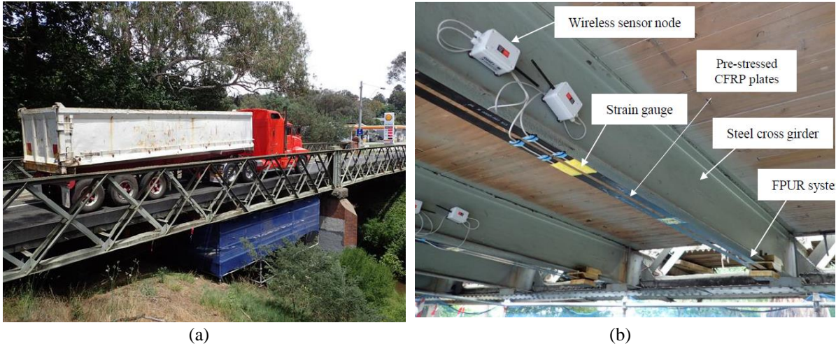
Figure 8. Diamond-Creek Bridge: (a) 42.5-tonnes truck loading before and after strengthening; (b) application of FPUR system on two cross girders (Ghafoori et al., 2018).
