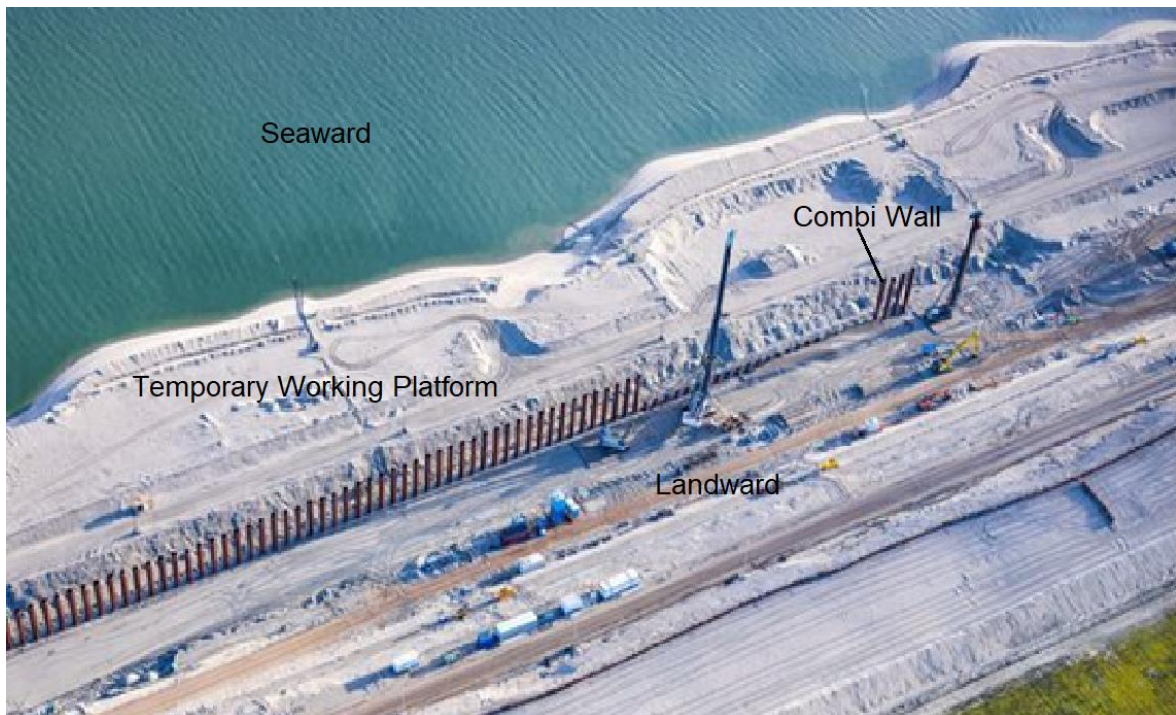
Figure 16 Installation of large diameter open-ended piles for a deep sea quay wall ( https://www.portofrotterdam.com/en/building-port/ongoing-projects )
