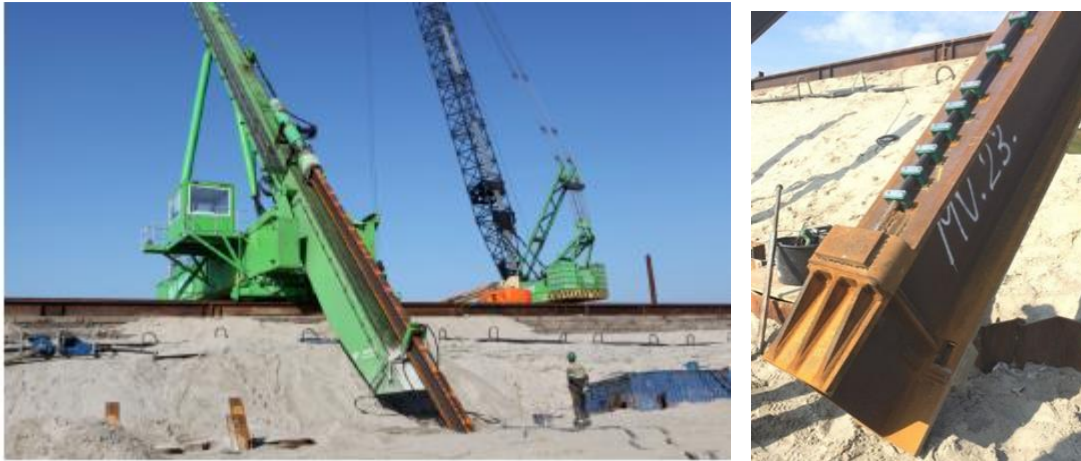
Figure 15 (a) Driving of an MV Pile (b) Pile toe showing grout tubes (Westerbeke 2021)
