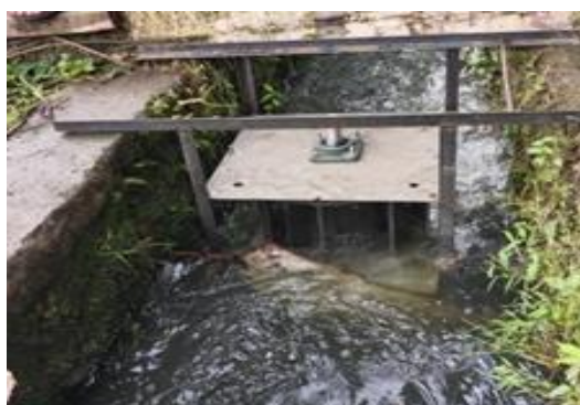
Figure 5. Turbine placed in a water line
