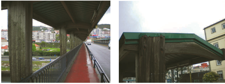
Figure 1.52 Examples of Use Classes from a road bridge in Spain (courtesy of David Lorenzo).
