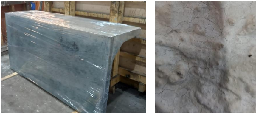
Figure 9-5 Retaining wall (left, wrapped in plastic) and surface cracks (right, unwrapped)
