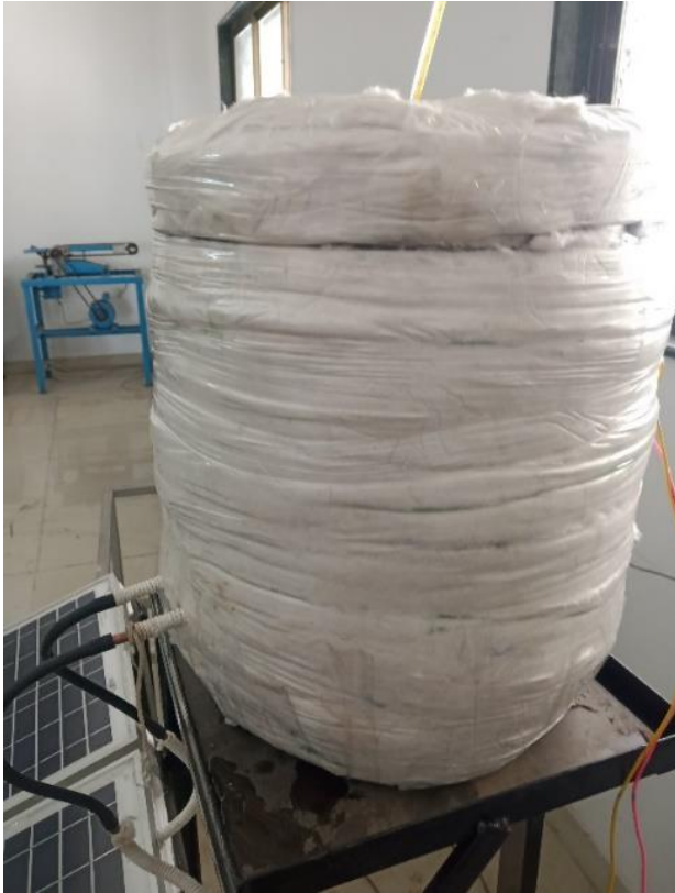
Figure 4 Image of Storage Tank
