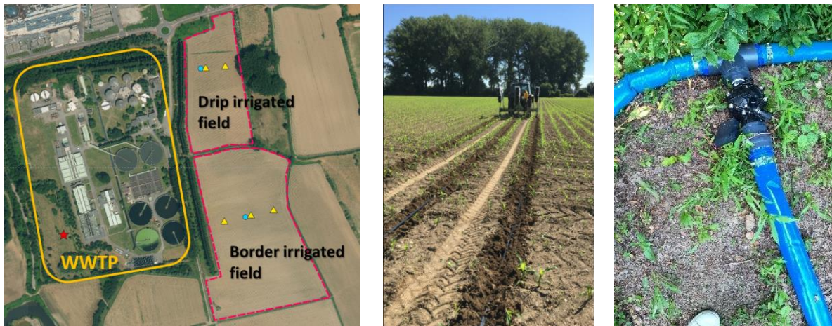
Figure 14: Overview of demo site (left), drip irrigation system installation (center), electro-valve regulating irrigation in each sector (right).
