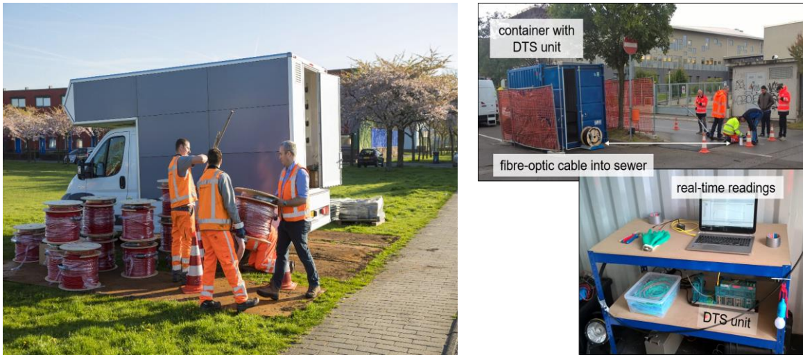
Figure 12: Mobile DTS unit with fiber-optic cables for detecting and localizing illicit connections in sewer (left) and container with DTS unit and fiber-optic cables (upper right picture) and actual DTS unit in container (lower right picture).
