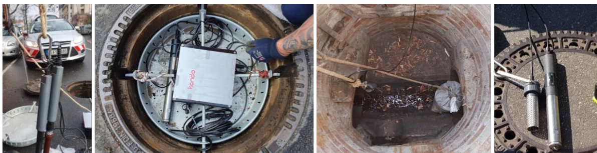
Figure 14: KANDO's smart unit and sensor (left), the EC sensor and logger (right) as well a sensor installed at a sewer manhole (middle).
