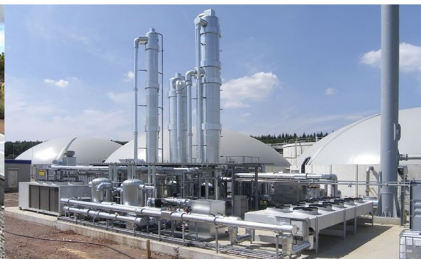
Kribi Thermal Power plant Source : Africa Energy Portal
