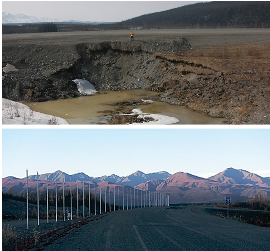
Fig. 7. Adaptive engineering to protect the Alaska–Canada Highway in a warming climate. A section that was especially prone to permafrost thawing and collapse (top; photo credit: Daniel Fortier), was rebuilt and fitted with thermosyphons to maintain the frozen state of the permafrost (bottom; photo credit: Fabrice Calmels).
