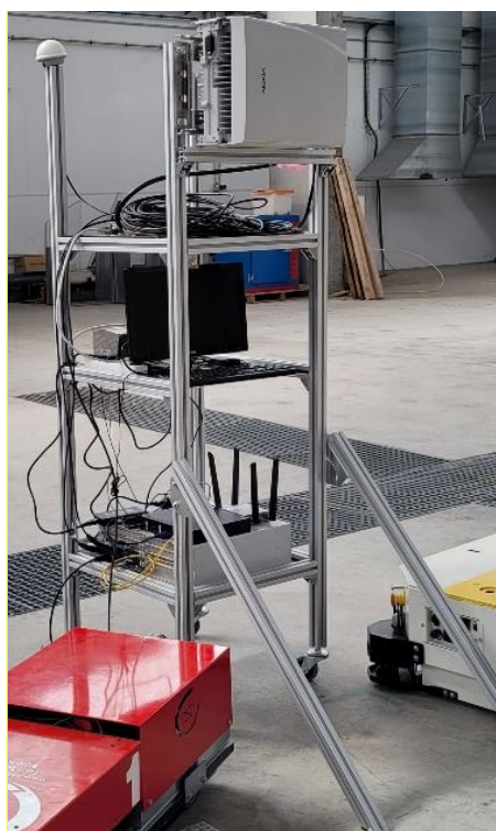
Figure 82: 5G base station
