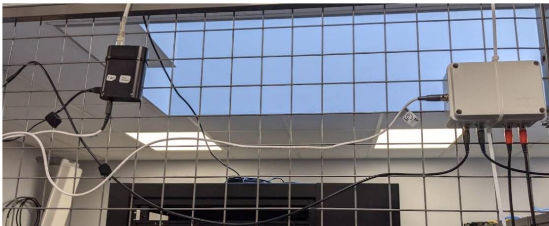
Figure 71: Heat sensors installed in iDR lab in Killarney.
