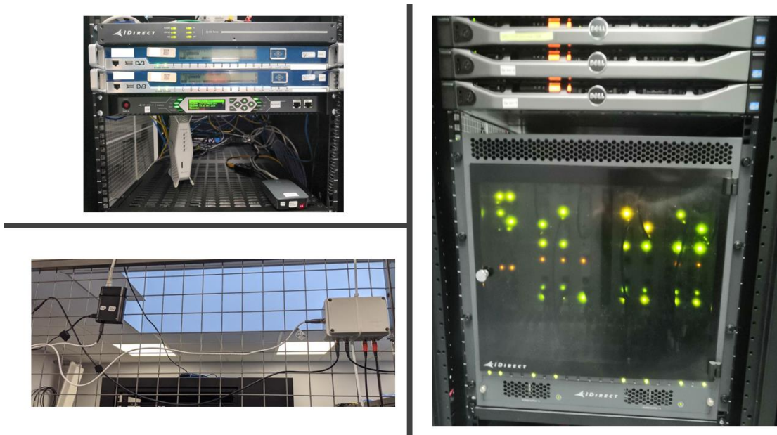
Figure 109: i) iDR Lab testbed including an iQ200, iQ Desktop, 9350 modems, IoT GW & Satellite Channel Emulators x2, ii) iDR Lab Testbed generic sensor used to measure temperature and humidity of the lab and iii) iDR Lab Testbed iDirect's 5G-enabled Velocity™ IGW hub
