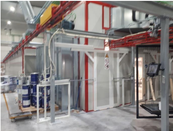
Figure 6 Coating area cabin (exterior)
