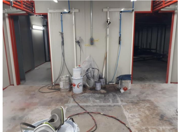
Figure 11 Finishing area cabin (interior I)
