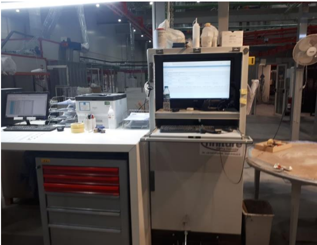
Figure 2 Process Control area
