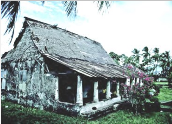
Sultan's House, 1986, before restoration. (Courtesy of Sir Ghilleain Prance, in Gardiner, B. G., 2008)
