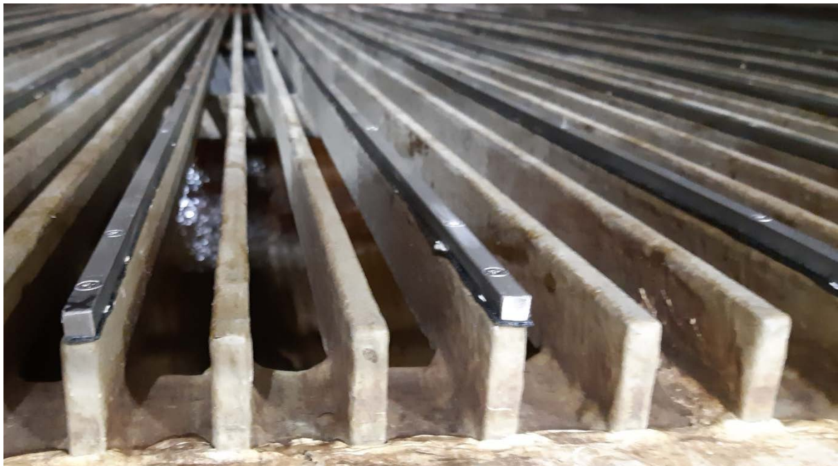
Figure 4.19 Illustration of installed electrodes on an old trash-rack within a hydropower intake (Source: Markus Auflager)
