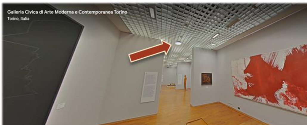
Figure 38. 5G Dot 4479 installation at GAM.
