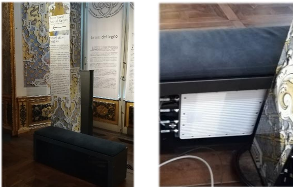
Figure 37. Indoor Radio Installation masked result and R4422 radio detail.
