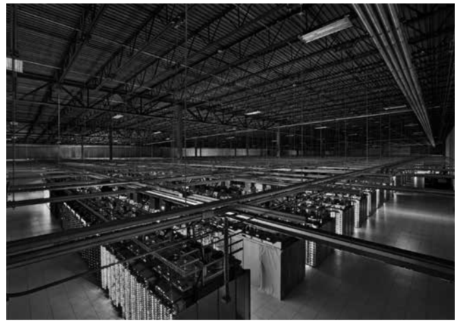
Google Data Center in Lenoir, North Carolina (USA), 2013. Both images served as founding documents and references for the research. Shown side by side, they confront an anticipative speculation to the implemented reality.
