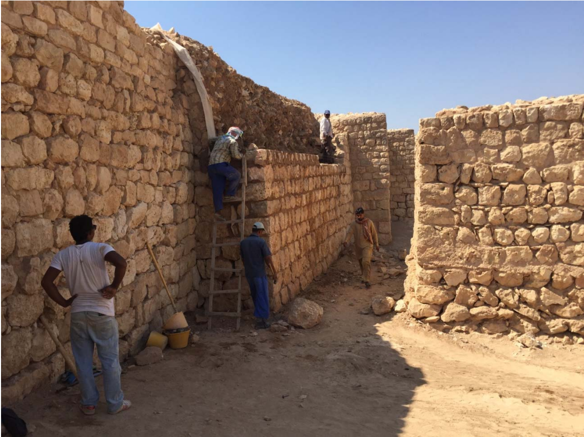
On 17 th November 2015, the wall was still under reconstruction as shown below.
