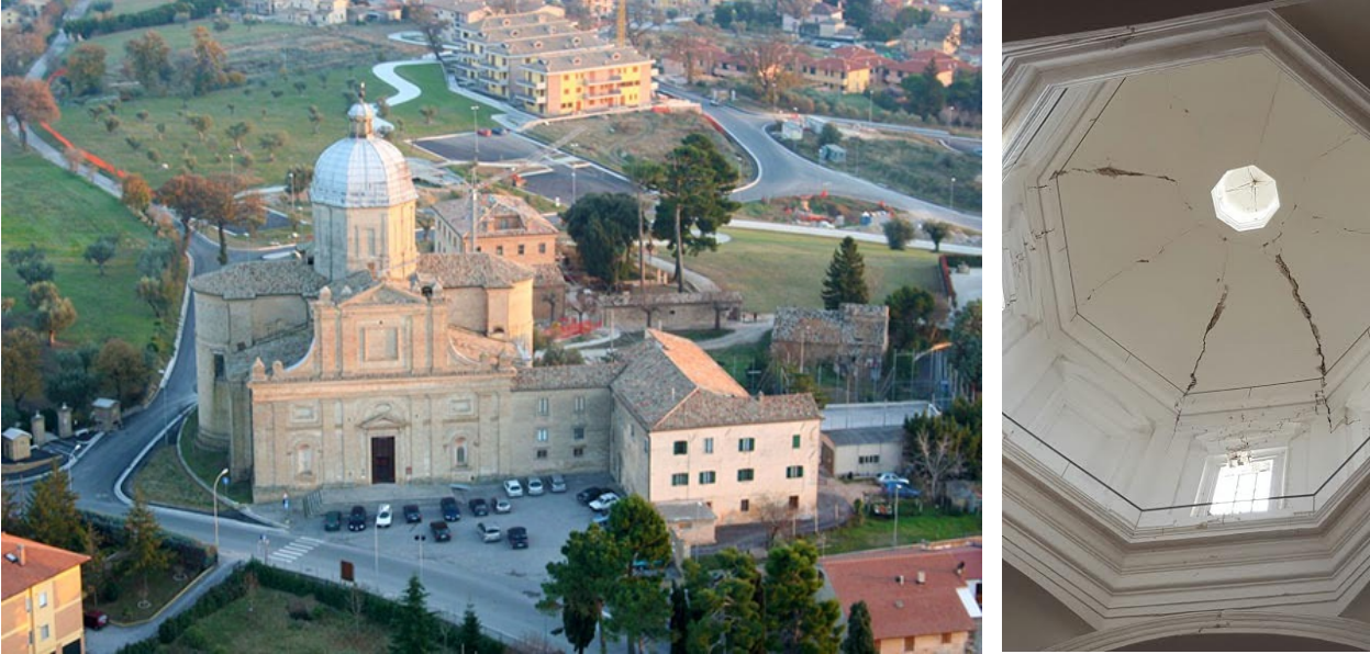
Figure 2: Aerial photo of the church of Santa Maria delle Vergini in Macerata before the 2016 earthquake (on the left) and the dome damaged in 2016 (on the right).
