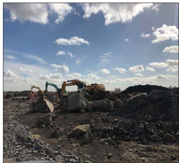
Figure 2. Site photograph of the large basalt rocks / floaters encountered at a land development site in Melbourne's north.
