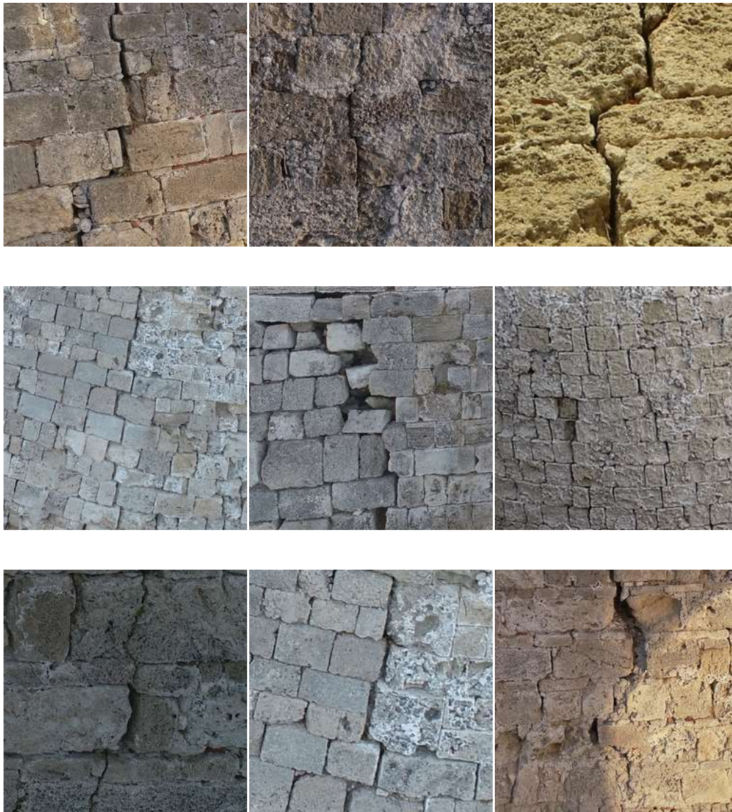
Figure 49: Images of the sites containing Cracks.
