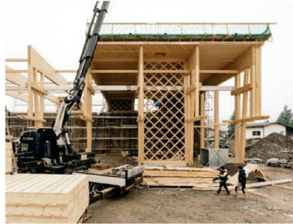
Figure 2. A finished and installed rhombus truss at the 'Rauch' hall. (Photo by Hanno Mackowitz).
