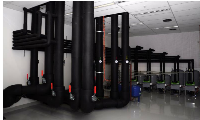
Cold and Hot water cooling
