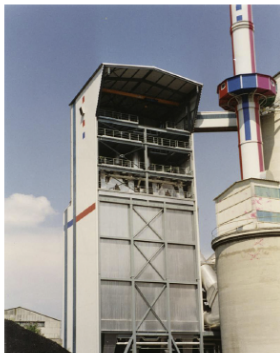
Fig. 4. Photograph of the lignite coke moving bed adsorber as it has been installed in 1994 (Rose and Brentrup, 1995); the photograph is used with the permission of Polysius AG, Beckum, Germany.
