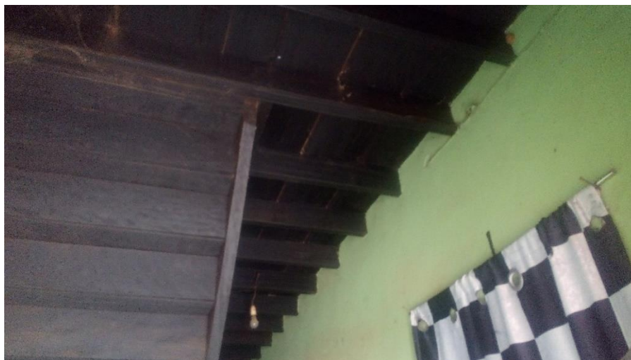
Plate 11: the timber slab that supports the load from the first floor which is painted for aesthetics purpose
