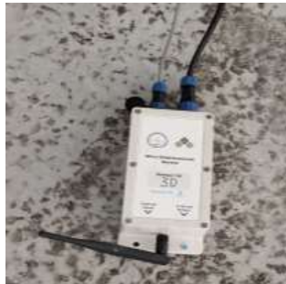
Figure 5. Bridge Monitoring System
