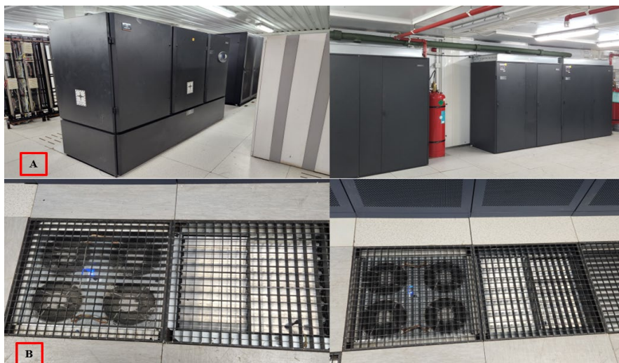
Figure 2: A – 35KW hvacs, B – Plenum Air Forced Extractor Fan on Raised Floor
