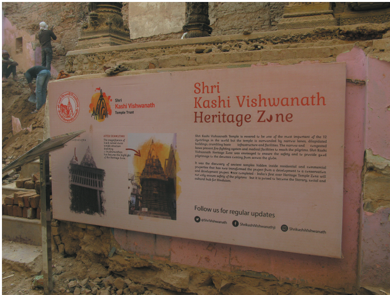
Figure 2. Work in progress and new sign board for the 'heritage zone', February 2019, Picture by author.
