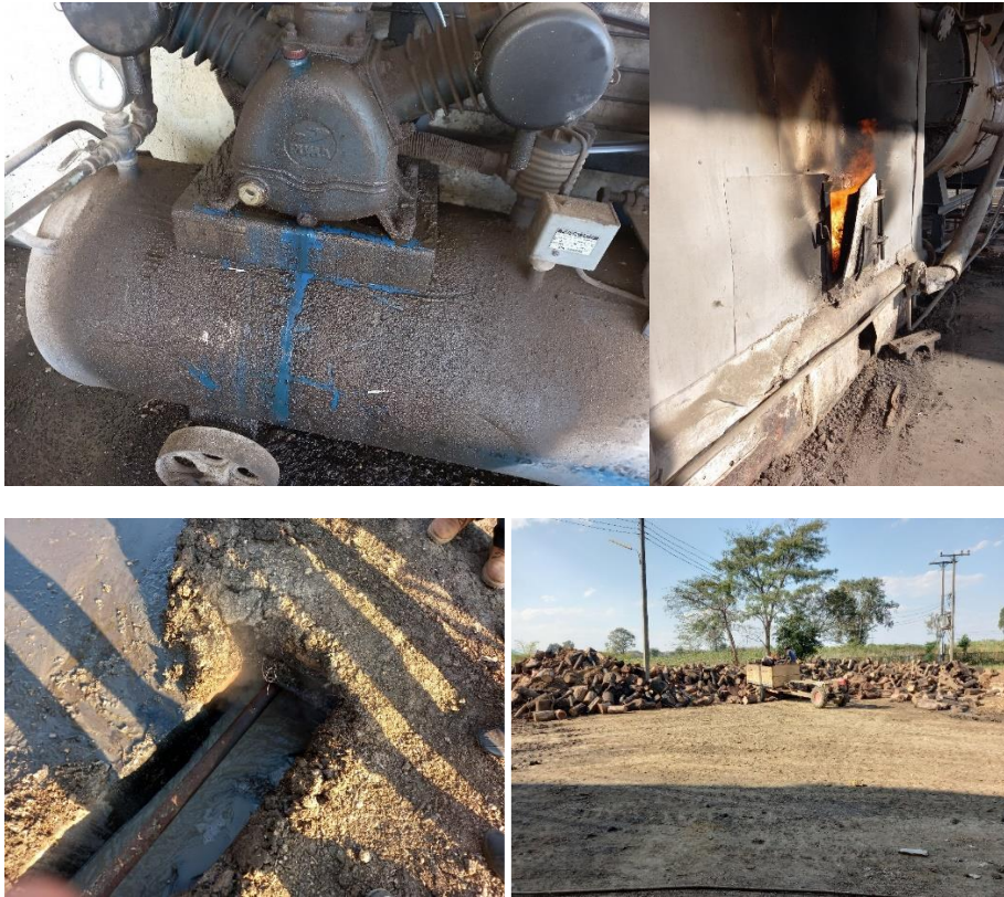
Figure 18 Inefficient air compressor using reciprocating pistons with oil leak (top left); inefficient wood boiler with leaking combustion chamber and poor thermal insulation (top right); condensates from the wood boiler that are not recovered or recycled (bottom left); and poor wood storage (bottom right).
