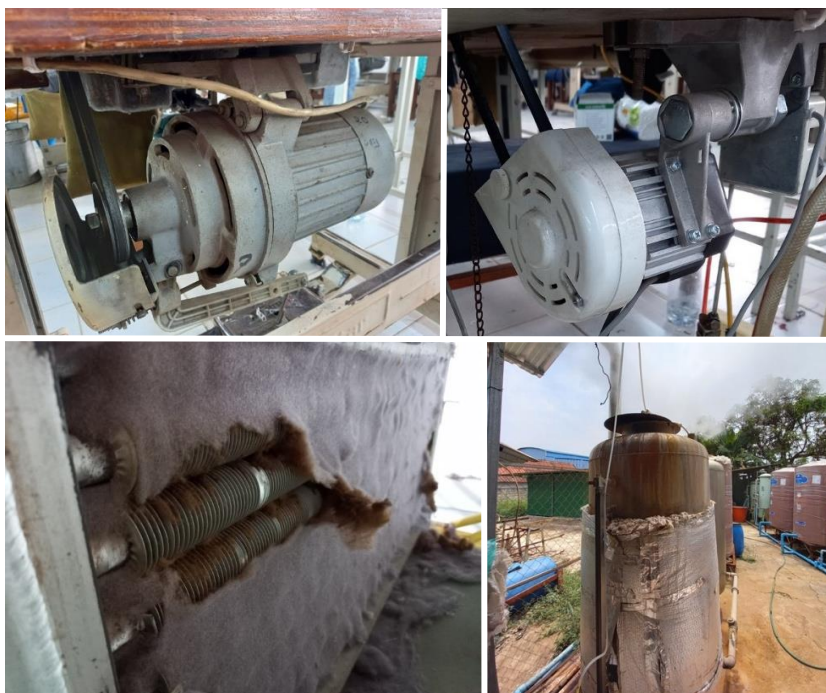
Figure 20 At the top: example of servo motors used in sewing machines in the Lao garment sector: inefficient clutch asynchronous motor currently used (top left) and improved motors that reduce energy consumption and minimize heat losses (top right). At the bottom: heat exchangers used by clothes dryers clogged with dust, thereby reducing the heat exchange efficiency (bottom left) and poor insulation of condensate tank (bottom right).
