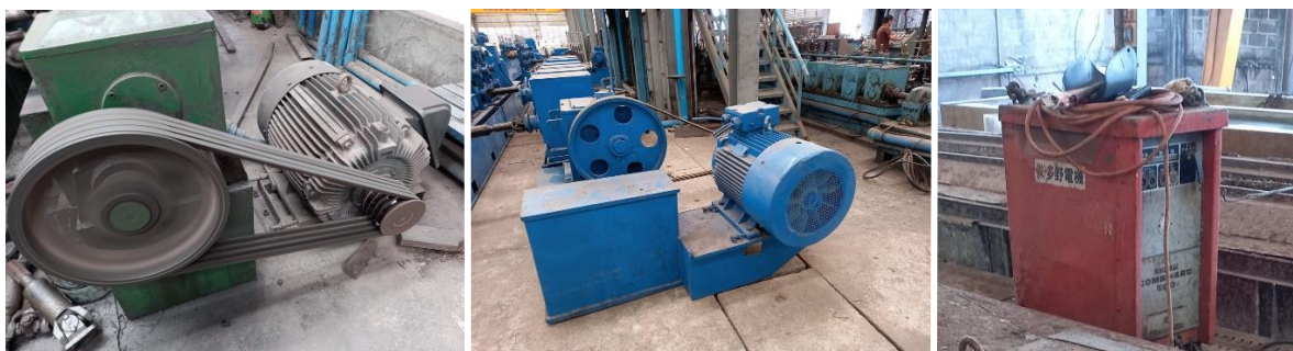
Figure 14 Use of inefficient V-belt transmissions (left) and electrical motors in tube-rolling machines (middle); and welding machines with conventional transformers including copper windings and iron core to raise voltage (right) in the steel industry.
