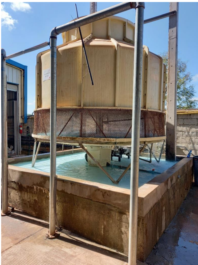
Figure 22 Chiller in plastics production facility that uses refrigerant R22, which is a hydrochloro-fluorocarbon (HCFC) refrigerant with high ozone depletion potential that has been banned in other countries.
