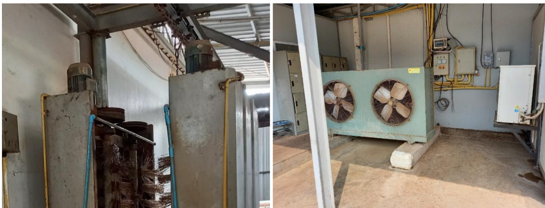
Figure 19 Inefficient AC motors (left); and inefficient chillers for cold rooms (right).
