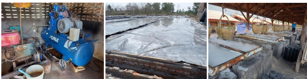
Figure 17 Inefficient air compressors using reciprocating piston technology with heat losses are used to pump brine (left); solar evaporation happening in open-air, leading to salt contamination and slow evaporation due to rain (middle); and inefficient open-air thermal evaporation process using coal or saw dust, creating air pollution (right).
