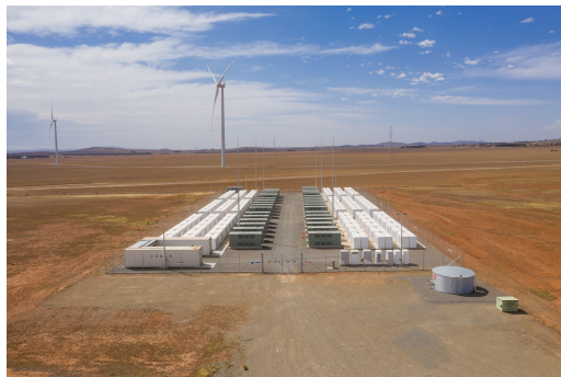
Hornsdale Power Reserve 129 MWh, 100 MW, 56 M€
