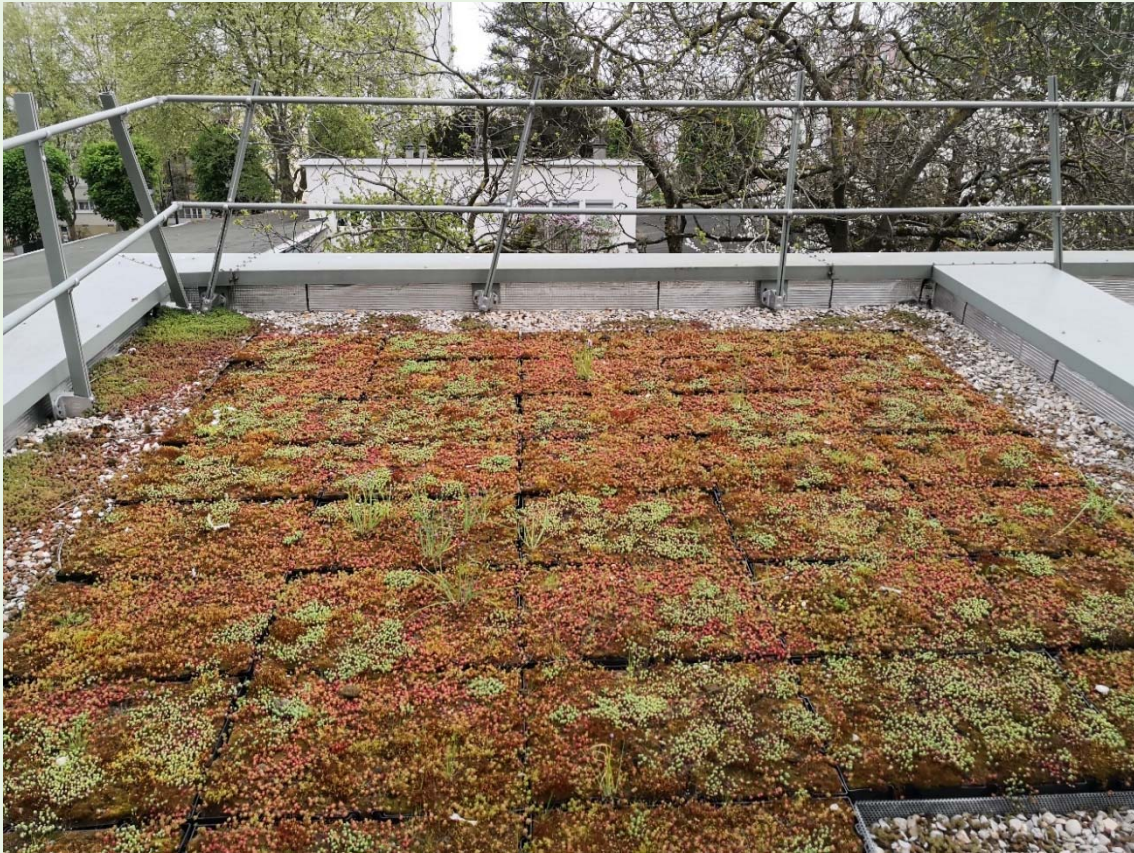
Some greening systems, such as these pre-cultivated sedum mats for green roofs, are often "copied and pasted" from one city to another. ©Marc Barra
