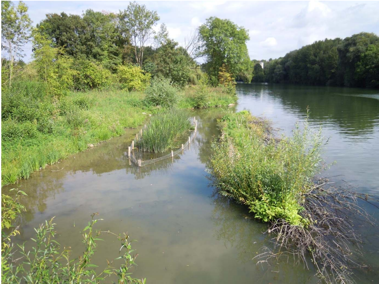
Ecological engineering techniques used to restore the banks in order to protect them from erosion, stabilise them and allow them to regenerate. ©Gilles Lecuir
