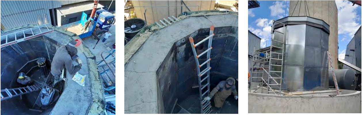
Figure 16: Internal reinforcements are removed (left). Pipes and bottom diffuser are implemented (center). Bottom supporting grid is installed. Top cover is pre-adjusted (right) [26-29/07/2022]
