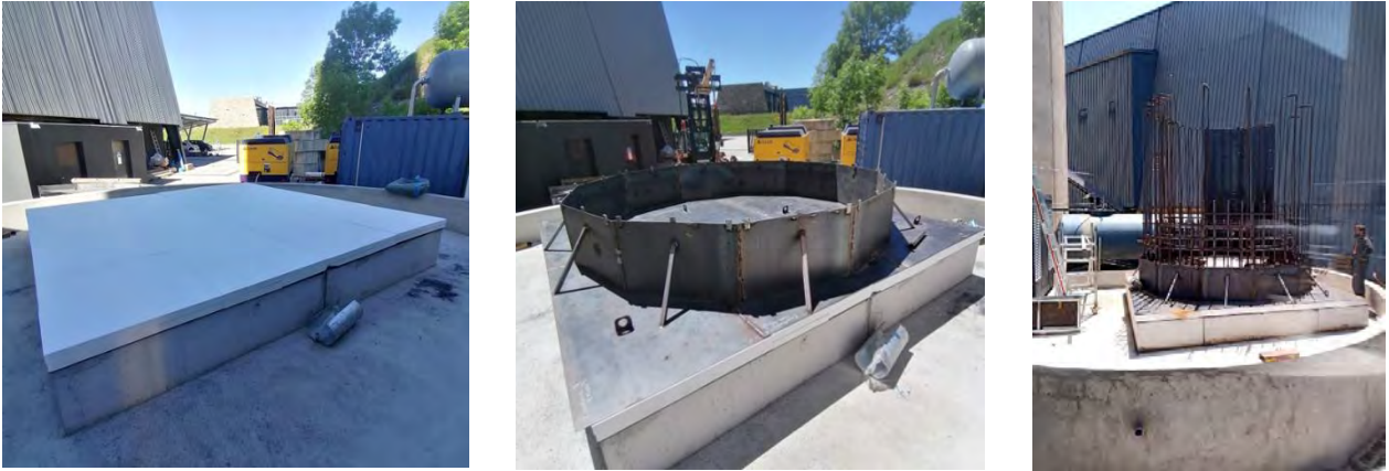
Figure 10: Implementation of insulation slab (left) and bottom formwork (center). Starting of construction of reinforcements for concrete wall (right) [13-17/06/2022]
