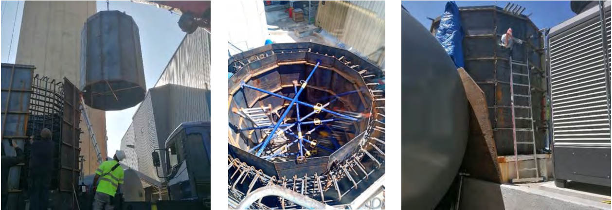
Figure 13: Installation of the inner formwork (left). Reinforcements of the formworks are set (center & right) [14-15/07/2022]
