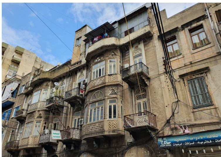
Buildings in al-Tell neighbourhood with informal construction on top floor. March 2020.
