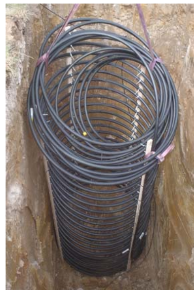
Figure 1: Earth basket spiral type heat exchanger installed at the IUT Civil Engineering, Student Laboratory (Bordeaux, France) pilot site.
