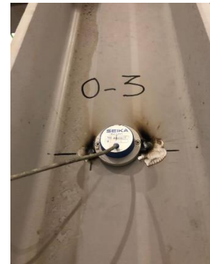
Figure 5 - Inclinometers employed for steel columns
