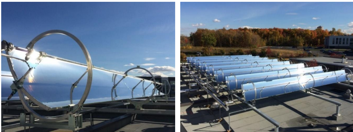
Fig. 1: Pictures showing one row of parabolic solar collectors (left) and the solar power plant (right).
