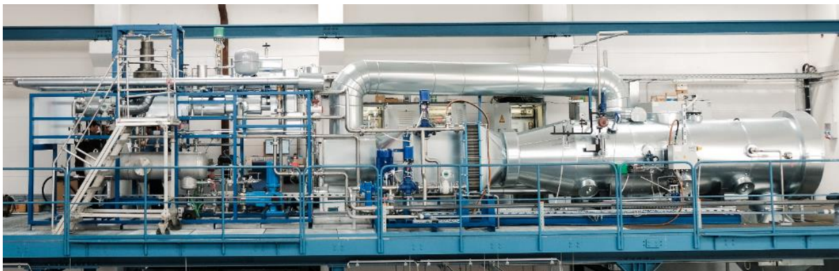
Figure 2: MicroRankine pilot SRC plant at the sewage treatment plant in Nürnberg
