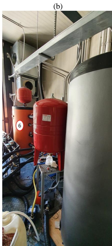
Figure 4: the testing rig at CNR-ITAE. (a) 1: LT storage; 2: HT storage; 3: piping connection manifold; 4: rack for acquisition hardware; 5: electric heating boiler; (b) 6: MT storage
