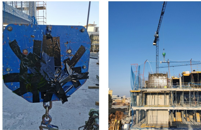
Figure 28: Sensor mounting on the crane hook #6 Barcelona
